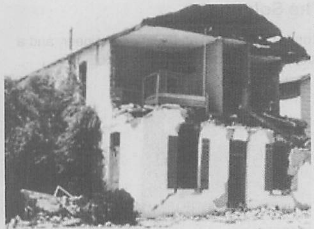
Figure 25 - The plaster-covered brick walls of this building collapsed during a recent earthquake.
